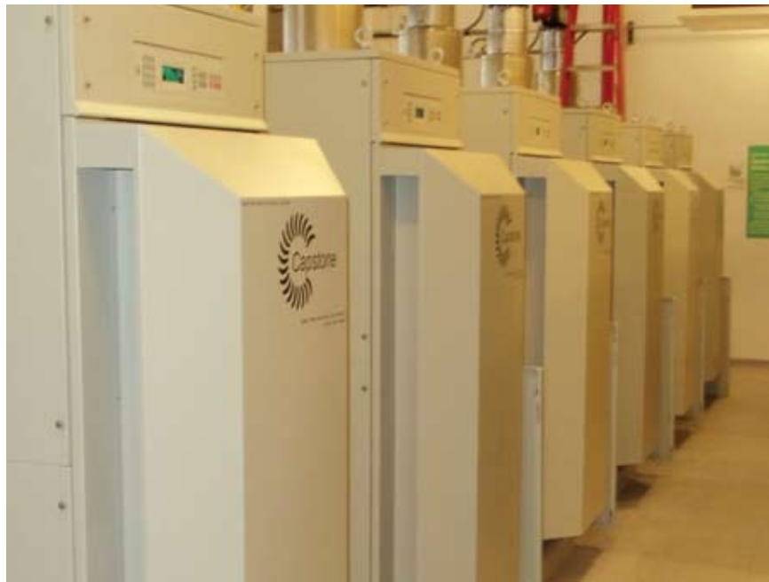
Twelve Capstone C65 Hybrid UPS microturbines are installed in Syracuse University's Green Data Center. The center is designed to use 50 percent less energy than traditional data centers.
