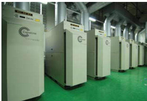
Ten C65 microturbines provide electricity and heating to a 44,520 m 2 apartment complex in South Korea.
