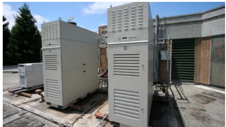
This county jail uses two Capstone microturbines for electricity and heating.
