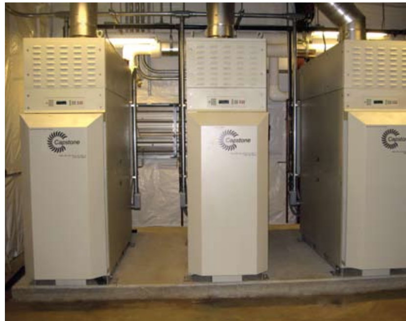
Commissioned in late 2009, the three natural gas C65 ICHP Capstone microturbines produce more than 80 percent of Davidow Hall's electricity and 100 percent of the building's heating and cooling.
