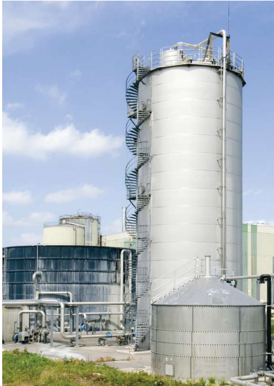
Capstone microturbines running on methane gas generate electricity and hot water for this paper mill in France.
