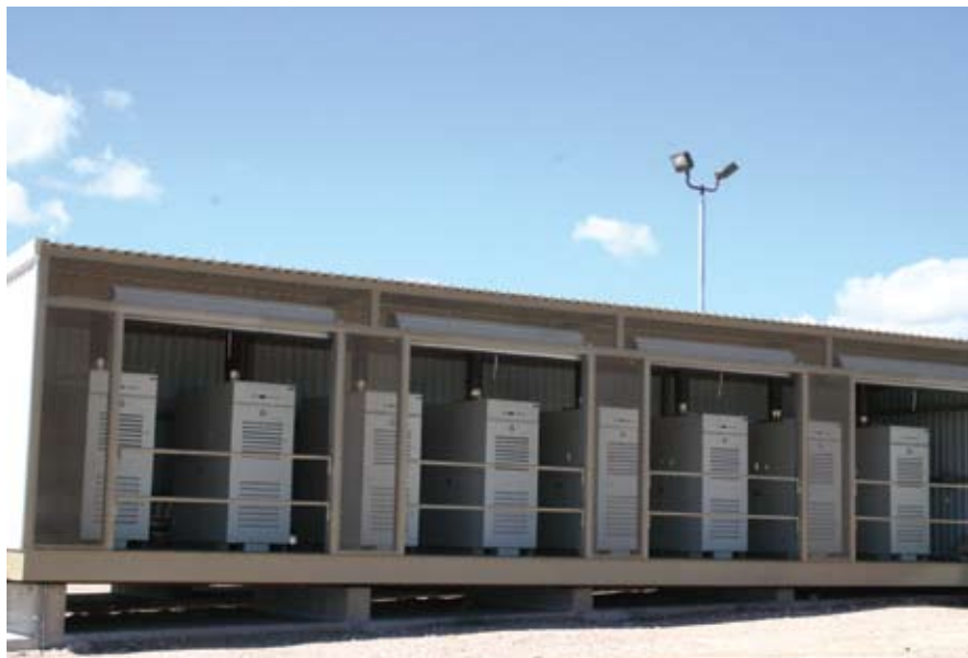
Fifteen 65 kW microturbines provide the primary power for this oil pipeline booster station in New Mexico.
