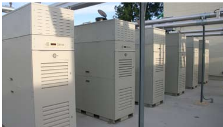
Six Capstone microturbines provide heating and on-site power at this Southern California college.
