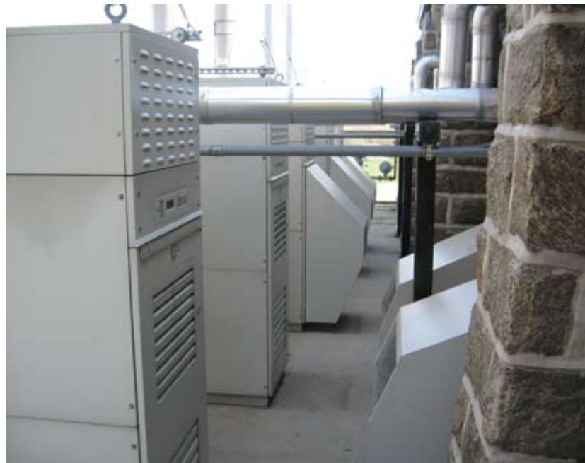
Capstone microturbines generate electricity and heating at Masonic Village, a 1,400-acre complex serving more than 1,700 residents since 1910.
