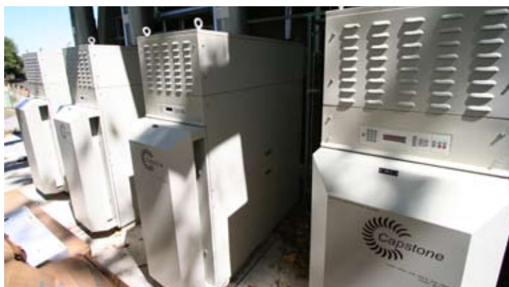
The pool at Foothill College is heated by four C60 kW Capstone ICHP microturbines.
