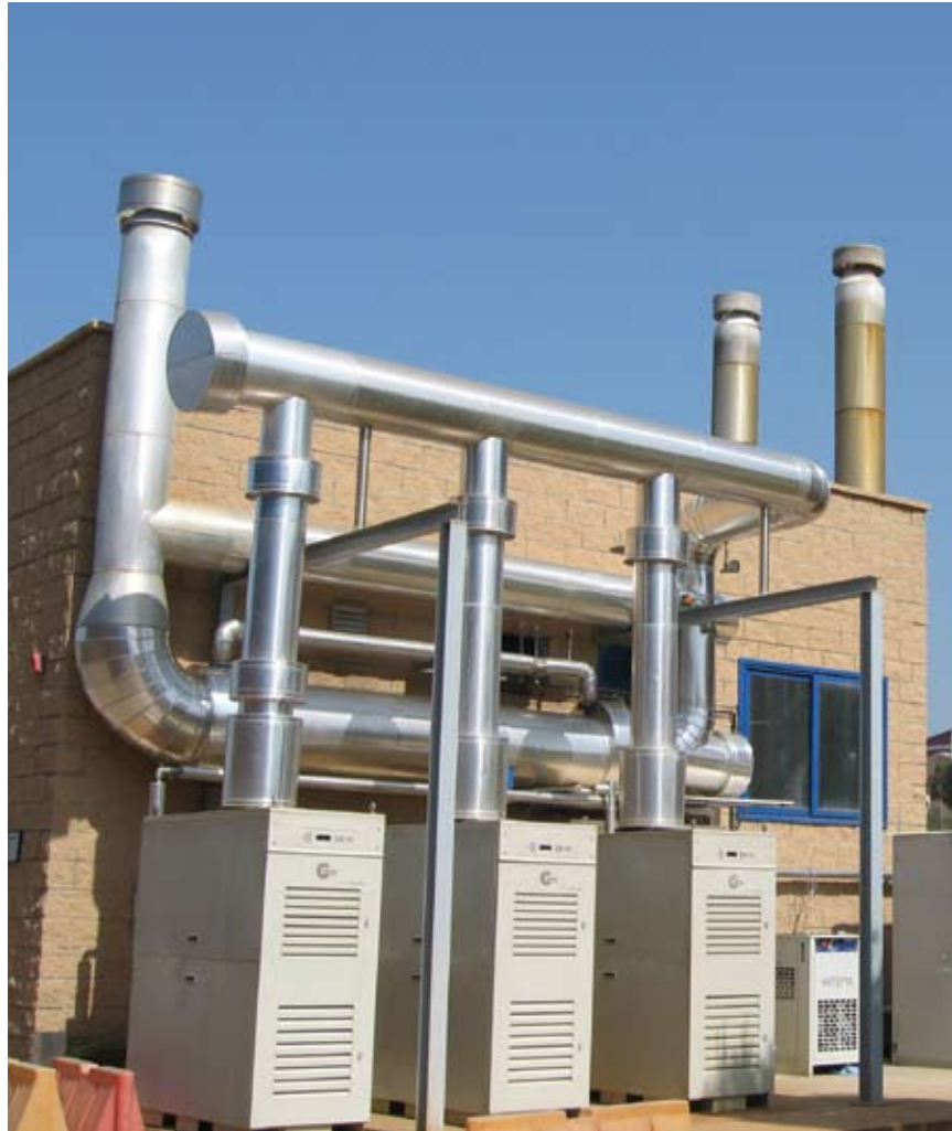
Three 60 kW Capstone microturbines running on biogas generate heat and power at Edar de Rubi WWTP in Spain.
