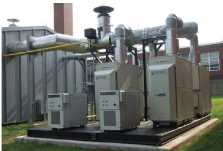
A PureComfort® 240M solution featuring four 60 kW Capstone microturbines provide cooling, heating and on-site power to East Hartford High School in Connecticut.
