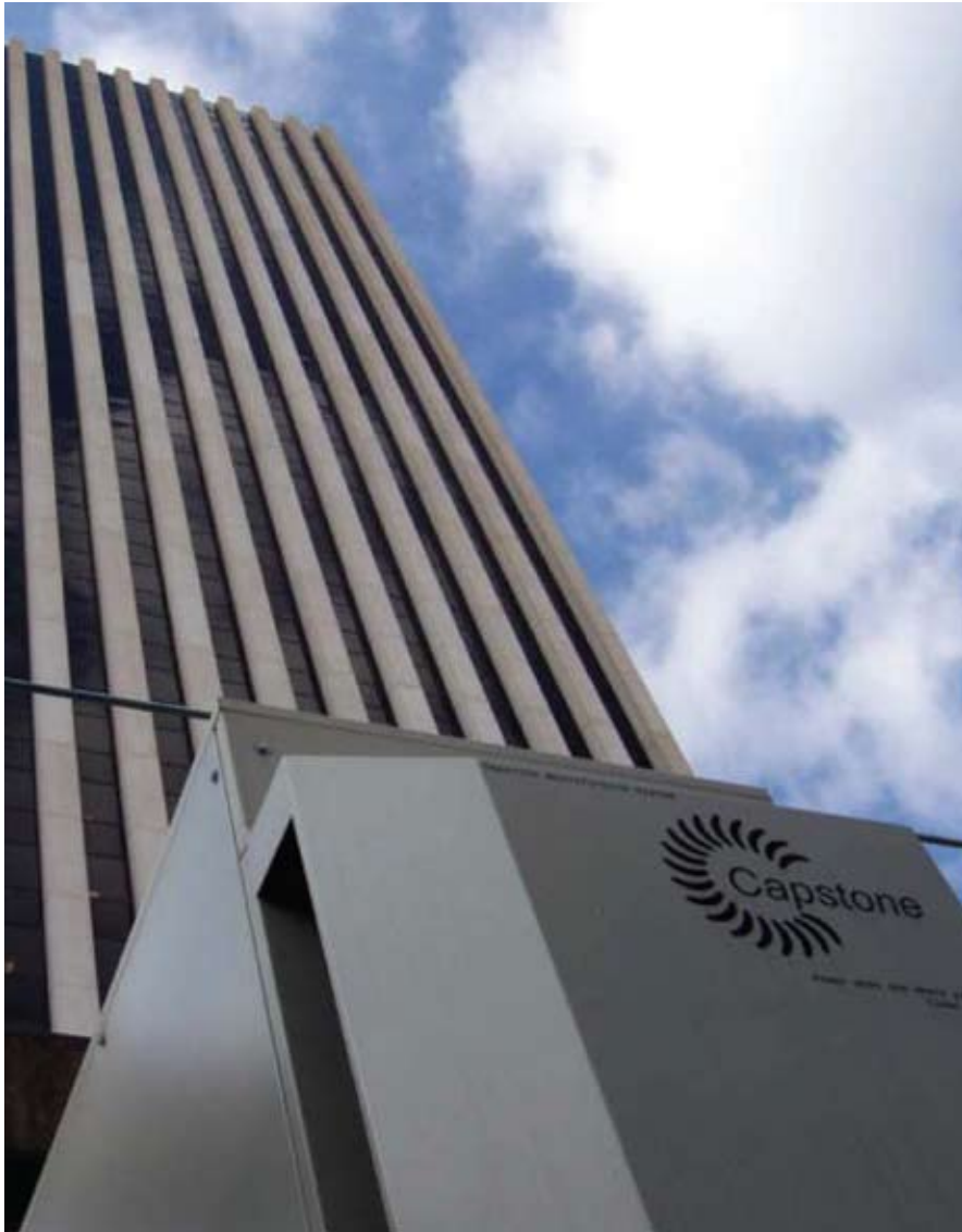
Six Capstone C60 microturbines assure power security at this downtown Houston site.
