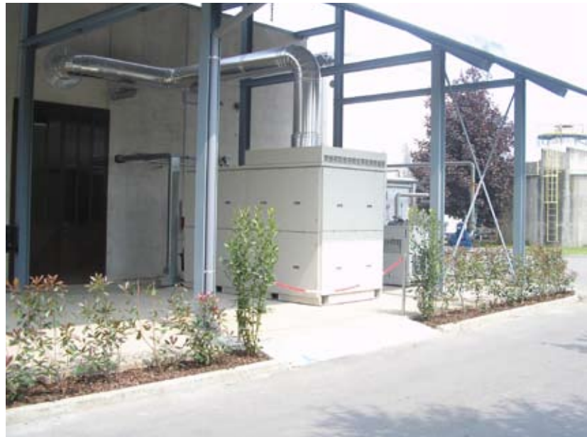
A single Capstone CR200 microturbine fueled by biogas, provides all the electrical power needed at the Cossato Spolina Wastewater plant in Italy.
