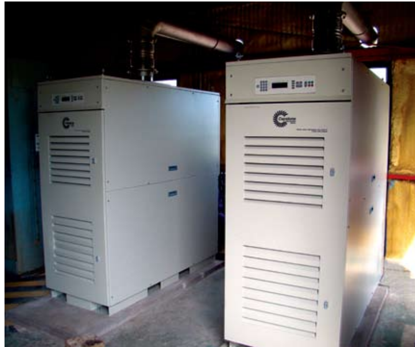
Eleven Capstone C65 natural-gas microturbines power compressors at this Bolivian pumping station.
