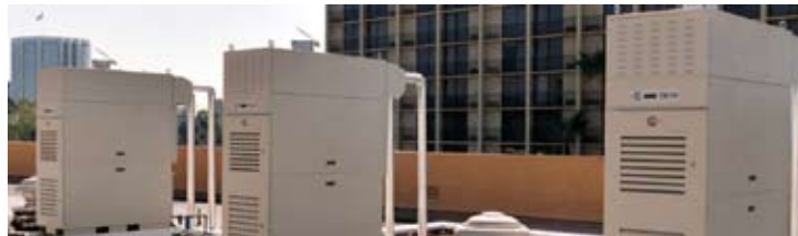
Capstone C60 ICHP microturbines provide heat and on-site power to the Atrium Hotel in Southern California.
