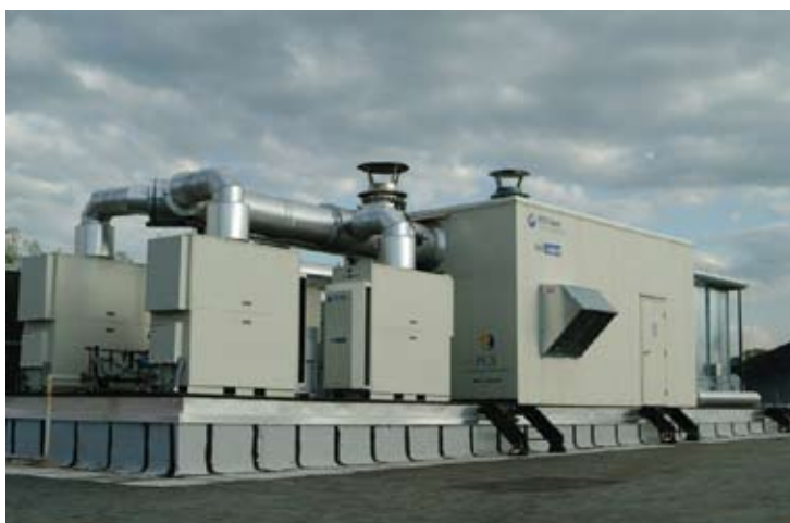
A PureComfort® solution featuring four 60 kW Capstone microturbines provide cooling, heating and power for this supermarket in New York State.
