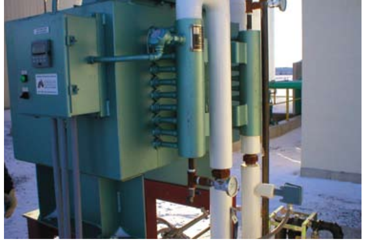
Cain Heat Exchanger for heat recovery from the Capstone microturbine.
